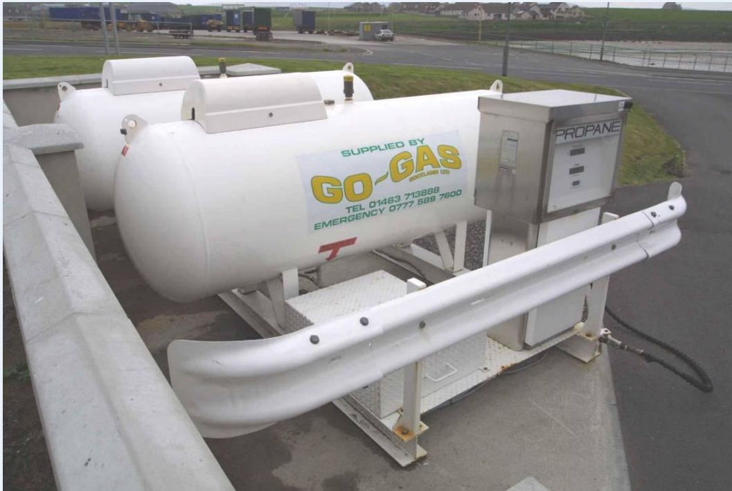
LPG tanks at the Stromness service station in Orkney
